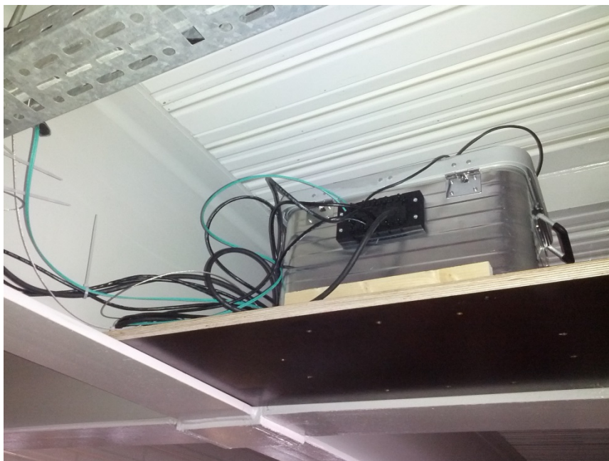
Figure 13: Communication hub placed under the garage's ceiling
