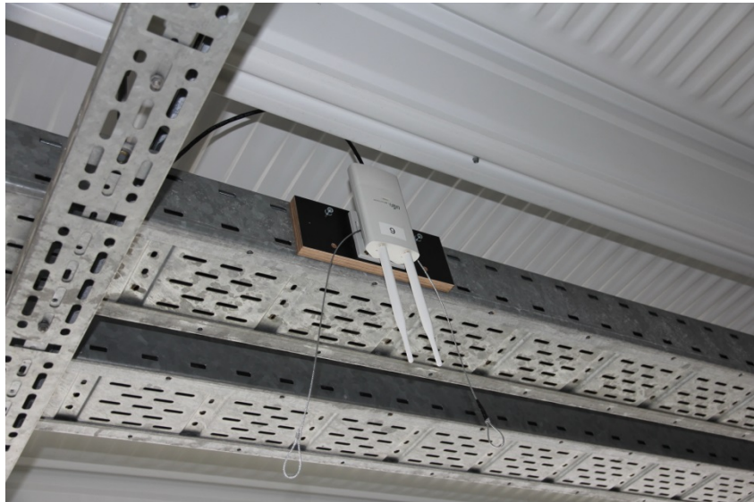
Figure 15: AP mounted on cable tray
