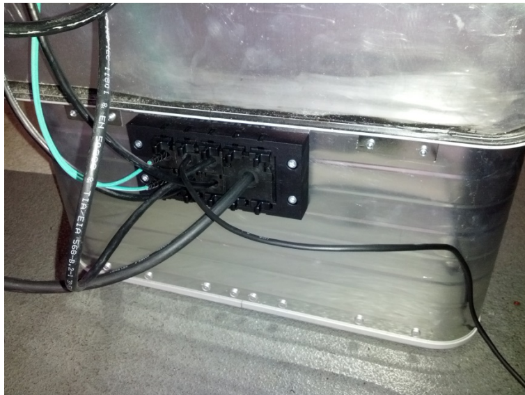
Figure 11: Cable feedthrough at indoor communication hub
